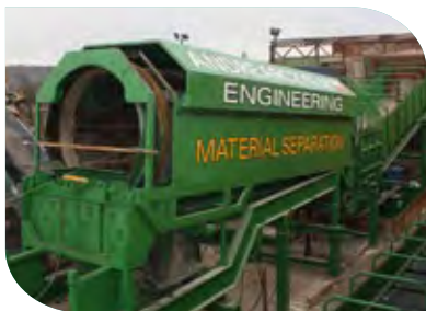
Our state-of-the art recycling plant
